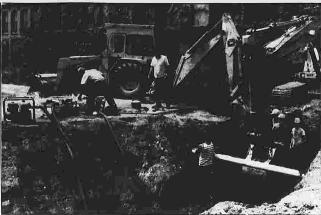
Workers from the town's Water Division and the Milton C. Beebe Constuction Co. repair a water line on Forest Street Friday after the line was accidentally broken by construction workers. The construction company is making improvements in the Cheney Historic District to be financed under a $750,000 bond issue.
